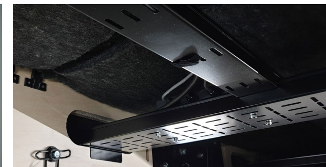
Cable-management within ceiling
